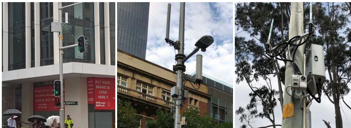
Figure 1: Typical Telstra Pole Mounted Small Cells
